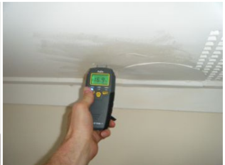
Old water stain
